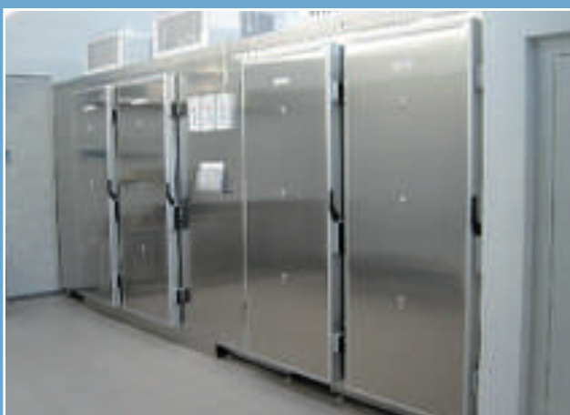
Gruppo celle per 15 posti salme, costituito da 5 vani, cadauno 3 posti, ognuno con proprio impianto / Group of mortuary refrigerators 15 bodies, divided into 5 rooms, each room 3 bodies, each room with its cooling unit
